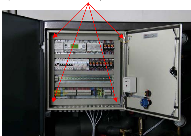
Photo: Fastening bolts of the switch cabinet
