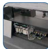
Plenty of room for cables, switches and power supplies in the generously dimensioned pedestal
